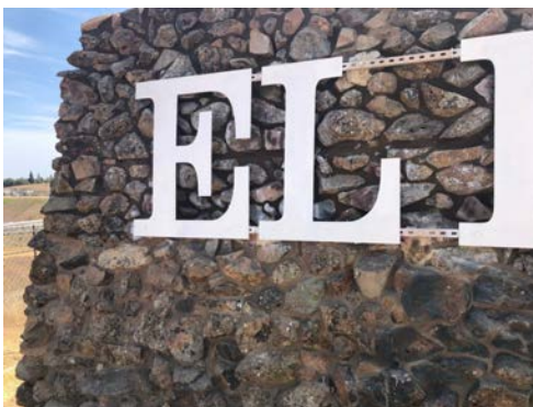
Wet mortar behind and above letters, dry mortar below. photo credit EDH Save Our Sign
