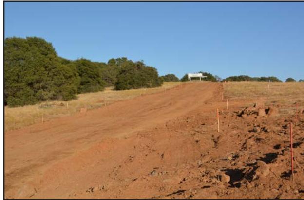
These two photos illustrate the grading on the new right-of-way for realigned Country Club Drive.
