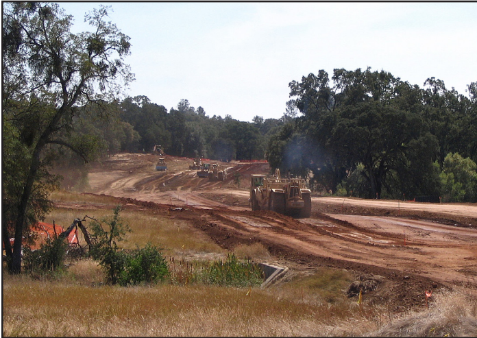
Earthmoving equipment preparing the roadway for Silver Springs Parkway, looking south along the right-of-way
