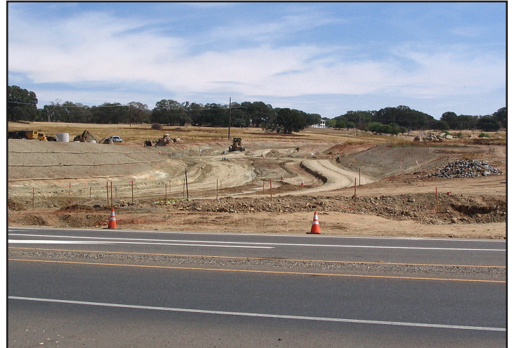
The realigned Sienna Ridge Road, looking south along the right-of-way from the Bass Lake Road intersection
