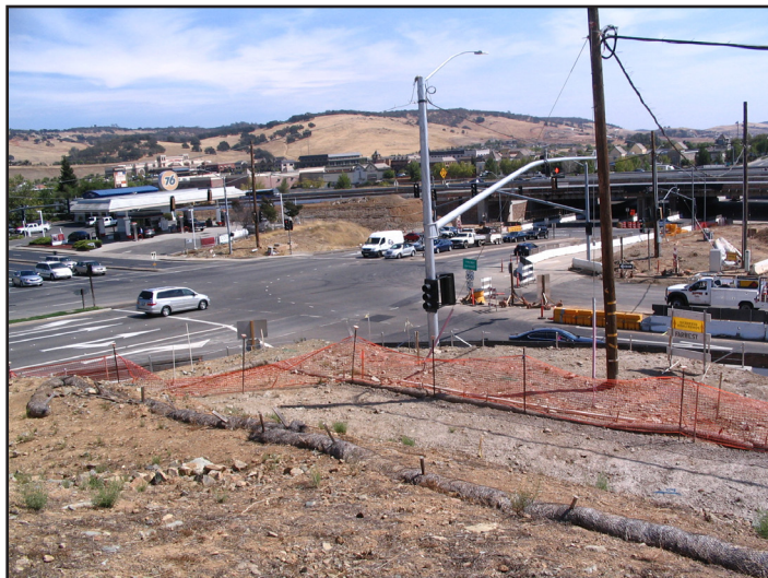
View of the new intersection created by the new on and off ramps at El Dorado Hills Boulevard
