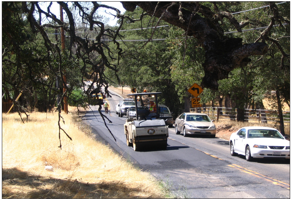
Road crew finishing up repairs to a dangerous pothole on Bass Lake Road
