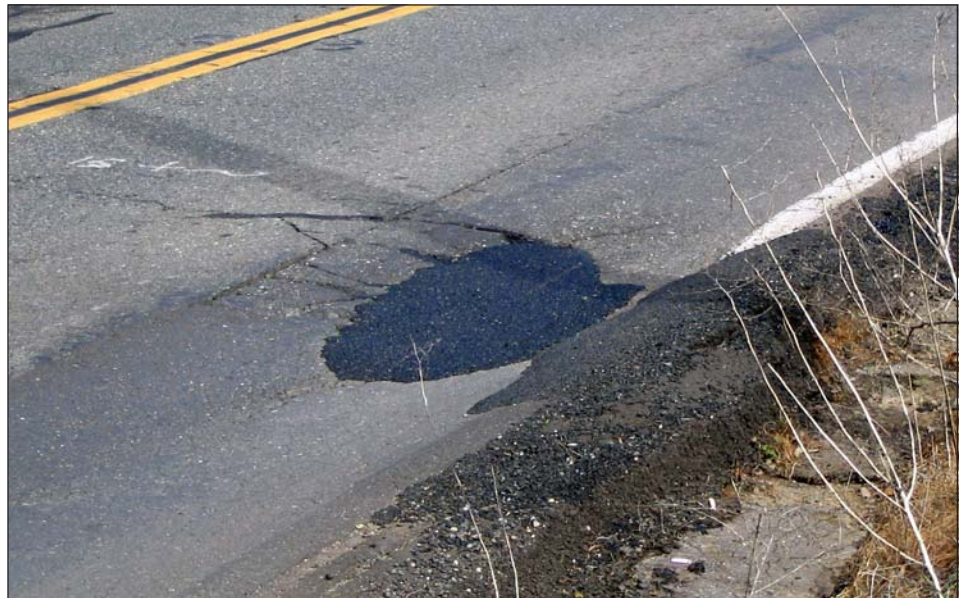
The new asphalt shows a pothole repair on the old part of Bass Lake Road near Magnolia Drive. Note that the new patch is on a previously rebuilt section of the roadway.
