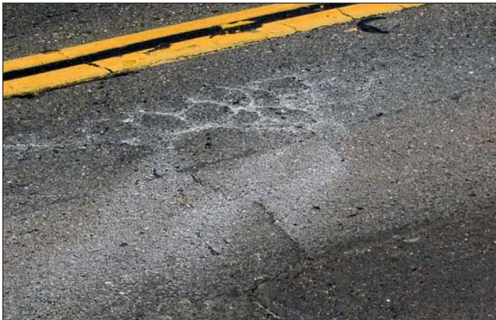
Example of water getting under the pavement and undermining the roadway on Bass Lake Road. The stains indicate that the substructure has probably softened due to water intrusion.
