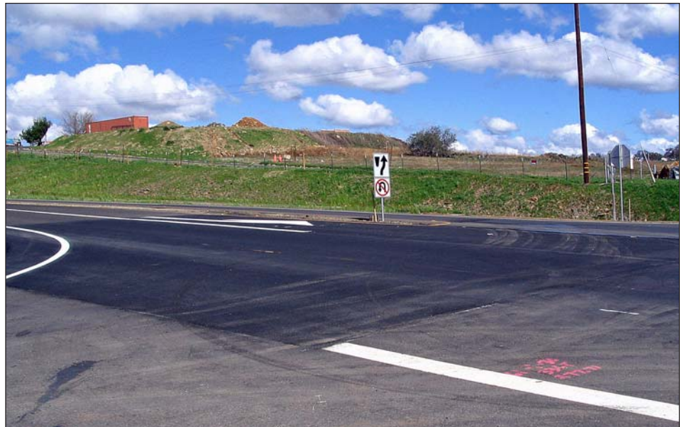
Leveled and repaved section of southbound Bass Lake Road at the intersection with Hawk View Drive on part of the new realigned road.
