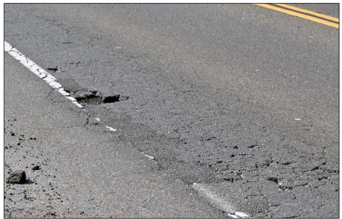
The beginning of a pothole on Bass Lake Road. Heavy vehicles have cracked the pavement and a chunk of pavement has been kicked out. Ongoing traffic will eventually create a pothole.
