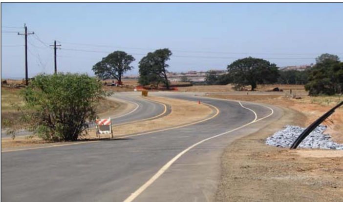
Looking westward to where the realigned Bass Lake Road connects to the new intersection with Serrano Parkway
