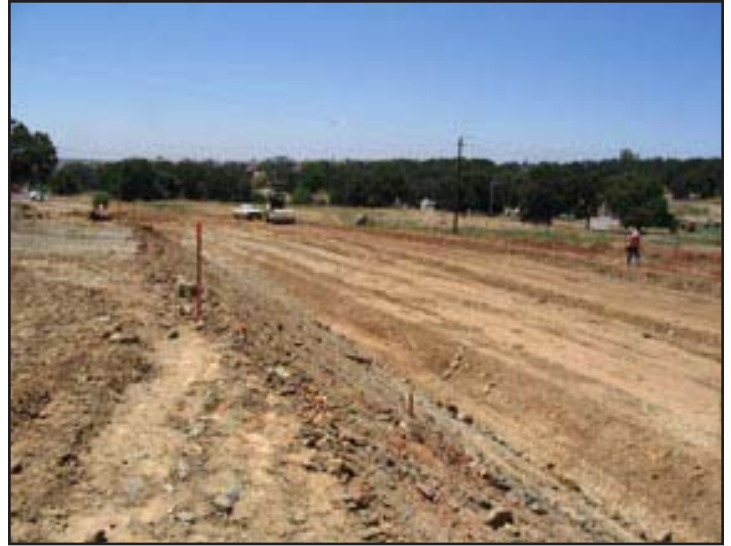
Looking south towards the new intersection where the realigned roadway will link up with Serrano Parkway
