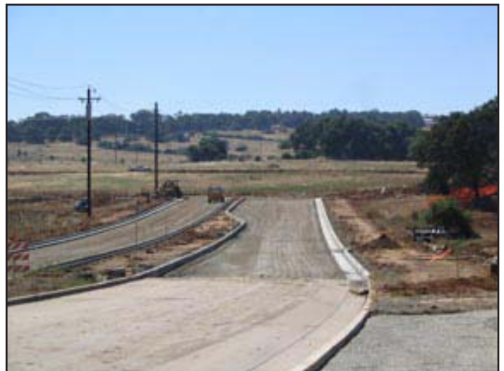
This photo shows the extension of Serrano Parkway to the new intersection where it will join with the realigned Bass Lake Road to provide easy access to Town Center.
