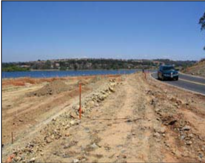
Looking north towards Bass Lake showing where the realigned roadway will meet the existing Bass Lake Road.
