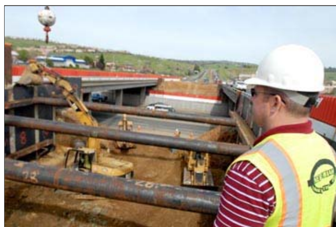
Chris Ellis, project manager with Nehemiah Construction looks out over workers clearing earth Democrat photos by Krysten Kellum
